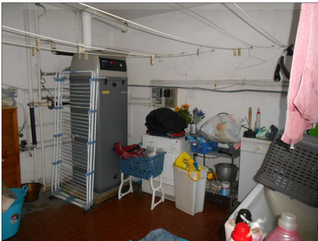
28 Piano seminterrato – Locale caldaia
